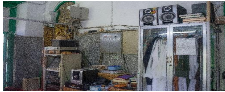
Figure 11. The sound system room
