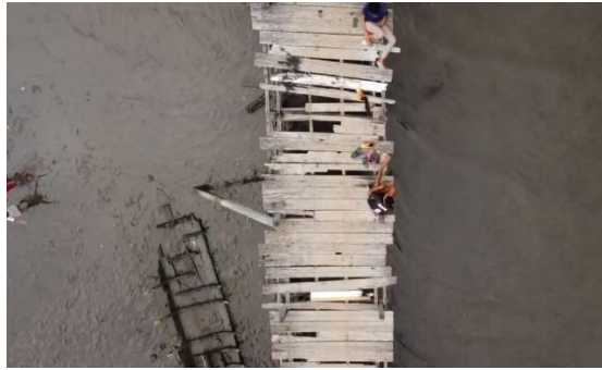
Picture 6. The condition of the dock in Warloka Pesisir Village
